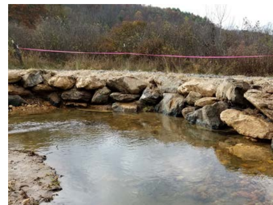
Figure 2. Large boulders and matting were used to stabilize the formerly eroding stream bank. The bog edge is immediately behind the pink flagging. Large gravel was laid down adjacent to the boulders to ensure the farmer could access his hayfield again.
