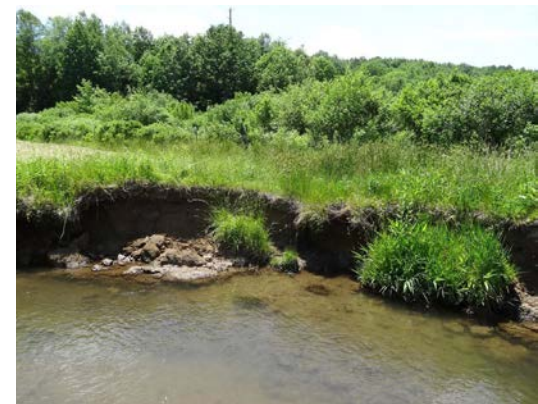
Figure 1. In this photo from May 2019, prior to the project, the streambank was eroding at a rapid pace and getting closer to the bog habitat with every large storm event. The shrubby area just beyond the sloughing streambank marks the edge of the bog habitat.
