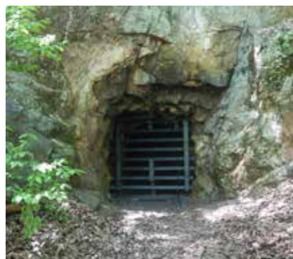
Entrance to a mine on Crowder’s Mountain State Park before and after gate installation (Katherine Etchison)
