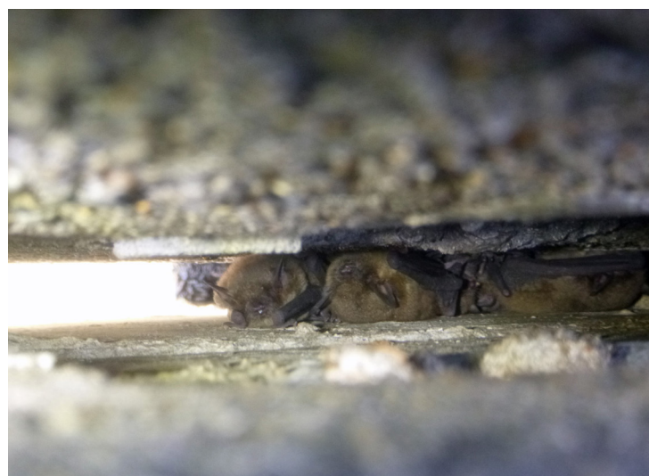
Gray bats roosting in the expansion joint of a bridge (Photo by Katherine Caldwell)
