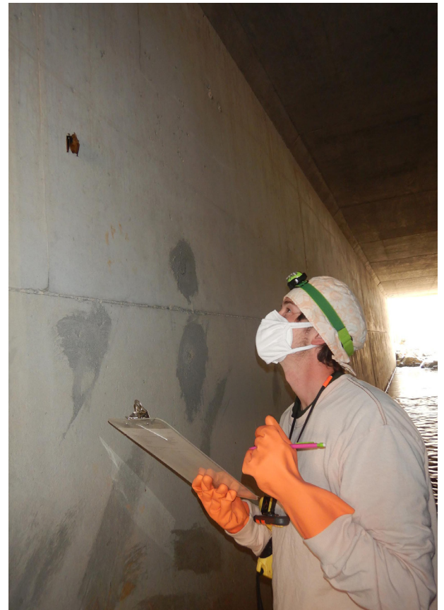
Wildlife Diversity Technician, Kyle Shute, inspects a hibernating tricolored bat in a Caldwell County culvert. (Katherine Etchison)
