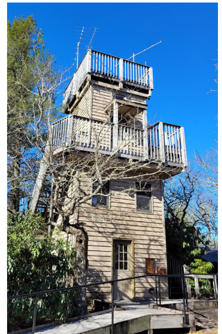
Directional antennas atop The Parry Family Tower at The Mountain Retreat and Learning Center (Christine Kelly)
