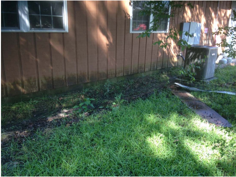
9. Visible Mold on Siding
