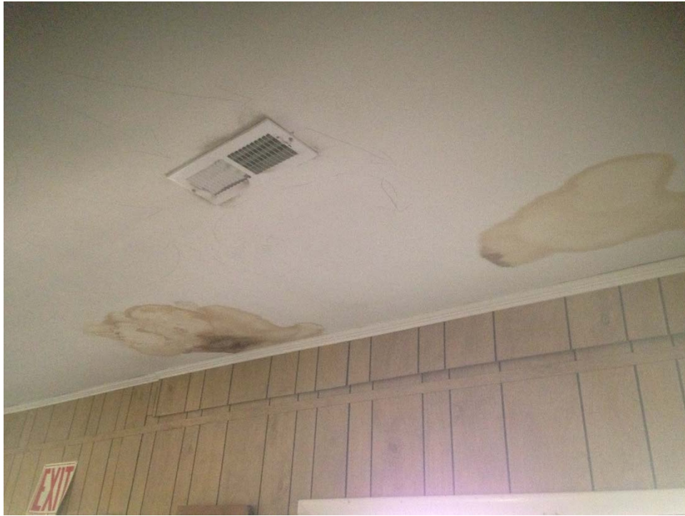
3. Stains on Ceiling
