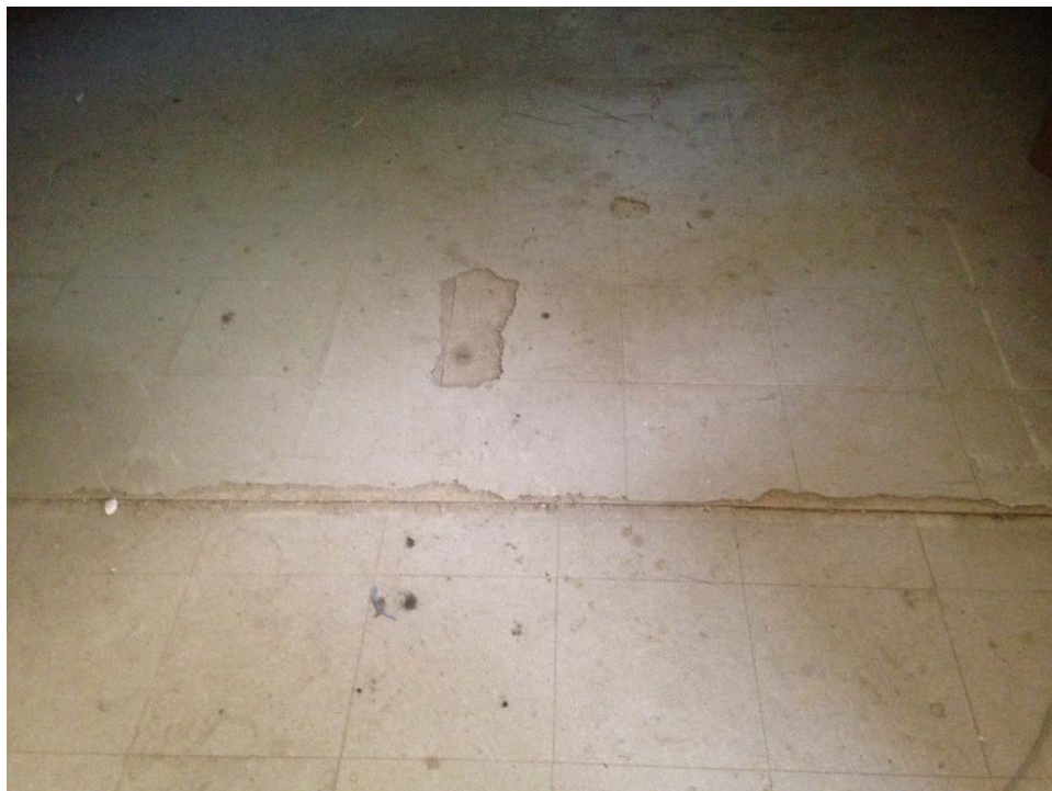
4. Damaged VCT Floor Tiles
