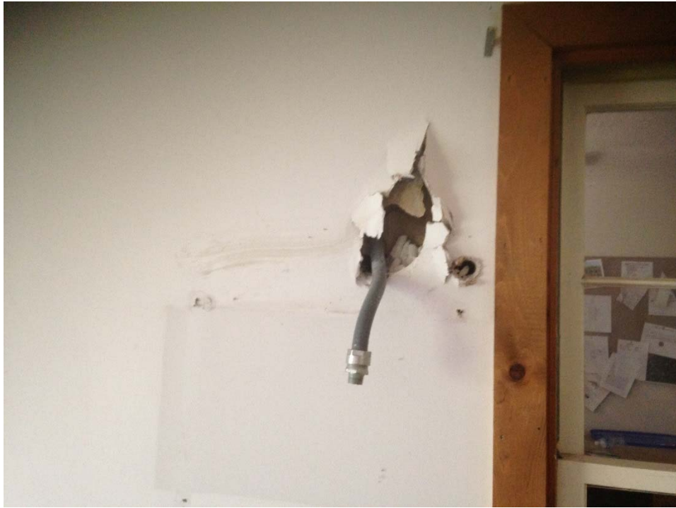
5. Exposed Conduit Protruding from Wall
