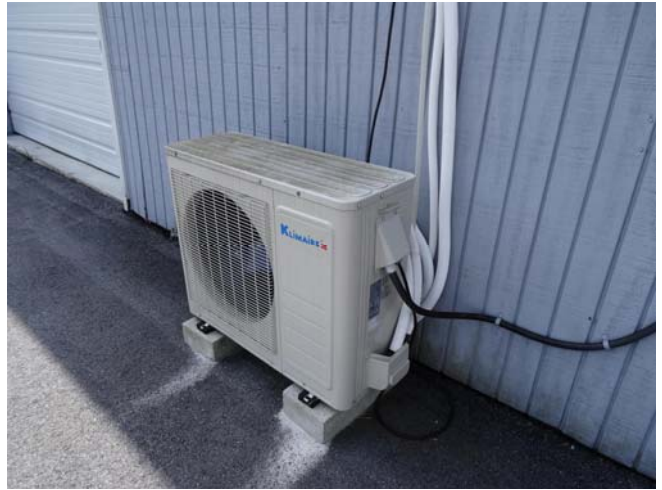
End bay mini-split AC pump
