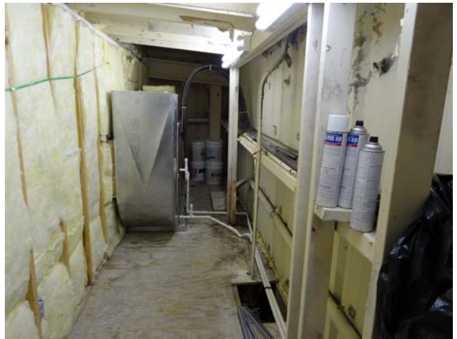
2 nd floor utility closet (air handler)
