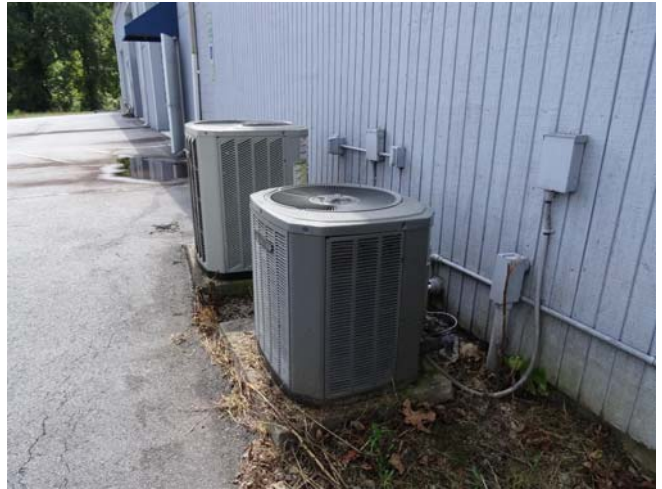
Office space heat pumps
