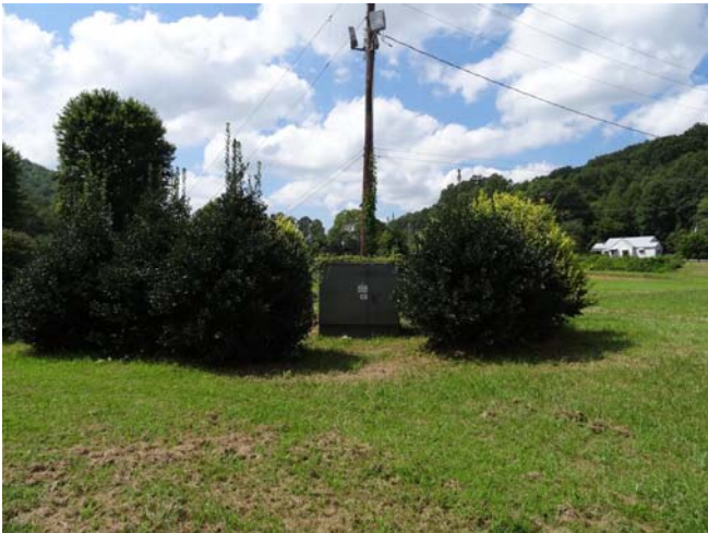
Transformer & Security Lights
