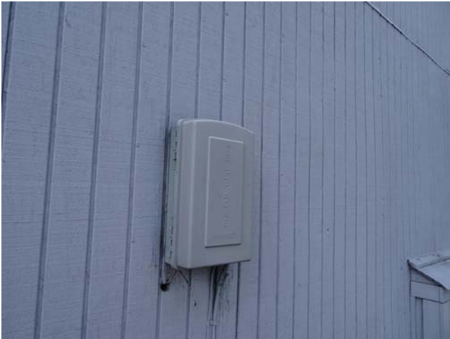
Telephone utility box
