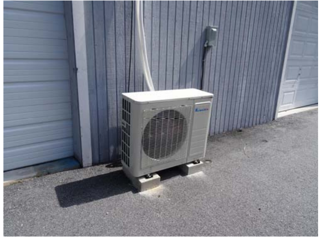
End bay mini-split AC pump
