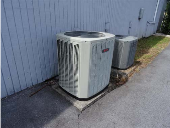
Office space heat pumps
