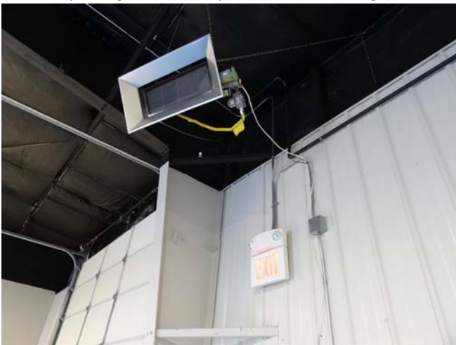
Center bay radiant heater (1 of 2)
