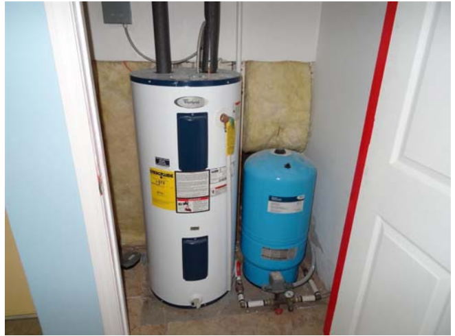
1 st floor closet (water heater & pressure tank)
