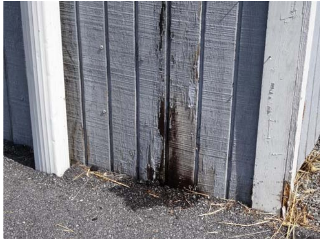
Water damaged siding
