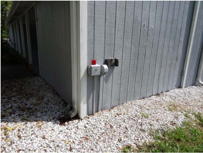
Septic lift station alarm
