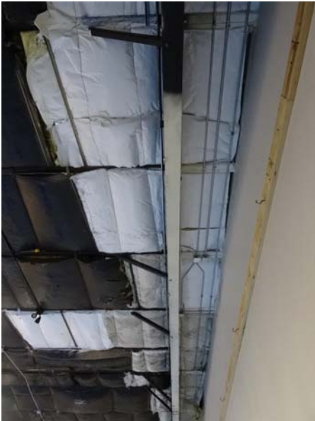
Center bay ceiling (insulation replaced after fire damage)
