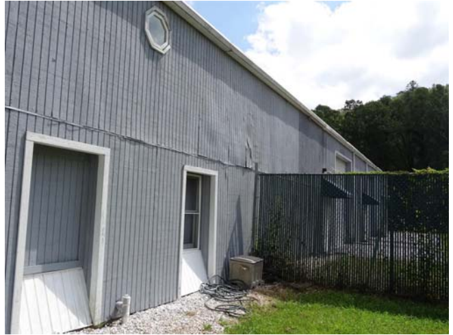
Damaged T1-11 siding
