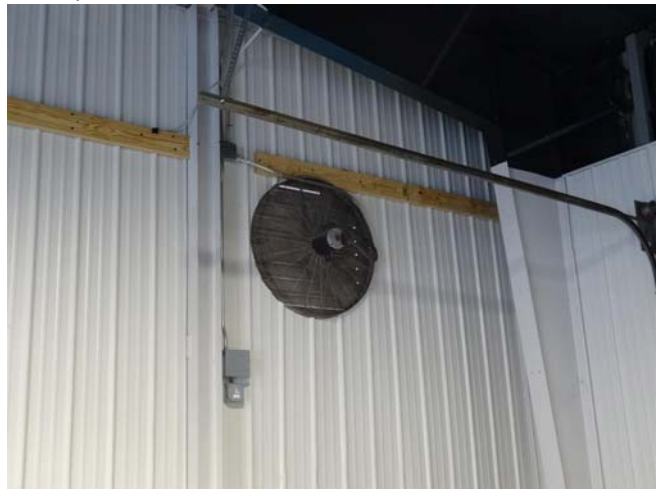
End bay exhaust fan (CO sensor)
