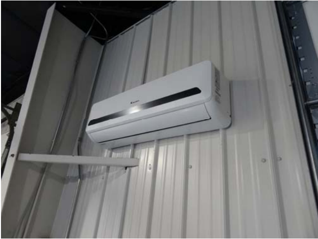
End Bay mini-split AC unit
